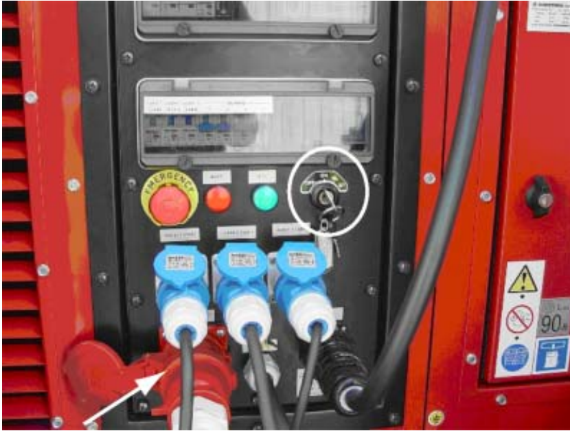
Image 3-2 Contact key and power cable of pump
